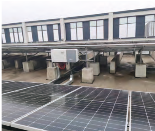
Photovoltaic Equipment on the Upper Floors of Sunan Smart City Science and Technology Industrial Park in Changzhou
