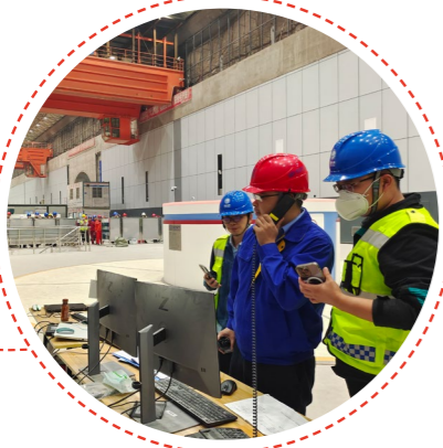
The on-site service team of DEC Machinery was conducting the trial operation and commissioning of the first unit
