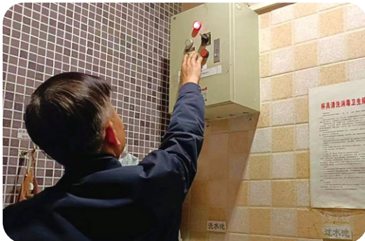
Investigation of Potential Safety Hazards in the Hotel
