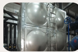
Air Conditioning Heat Recovery Project
