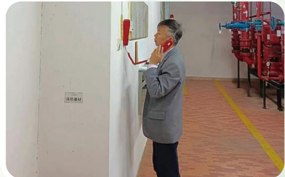
Hotel Fire Facilities Maintenance
