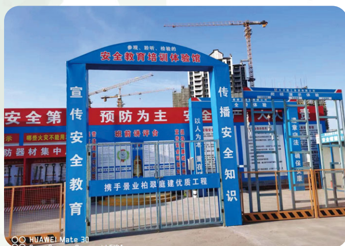
Production Safety Experience Zone
