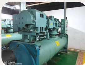
Central Air Conditioning Maintenance
