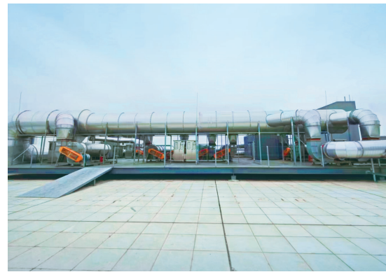
Upgraded Emissions Treatment Facilities 升級後的廢棄處理設施
