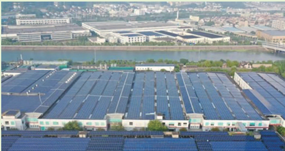
Photovoltaic Power Generation System
