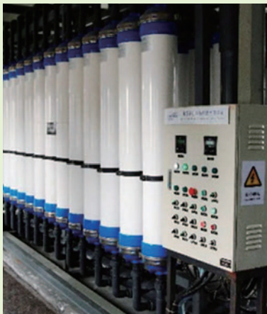
Ultrafiltration and RO Membrane Treatment Technology
