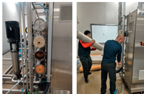
Membrane Treatment Unit for Water Purification System
