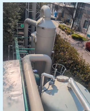
Exhaust gas two-stage spraying treatment device
