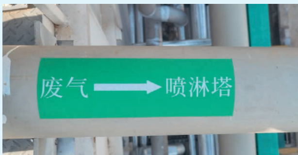
Waste gas collection pipe
