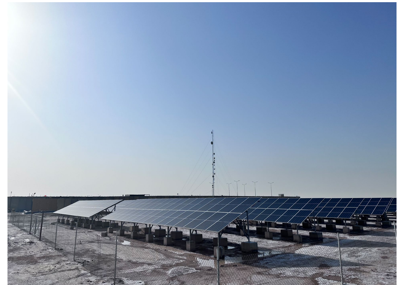
KEBL Camp Oilfield Photovoltaic Power Station Project
