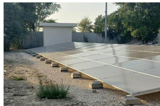
Naimat POD Solar Project
