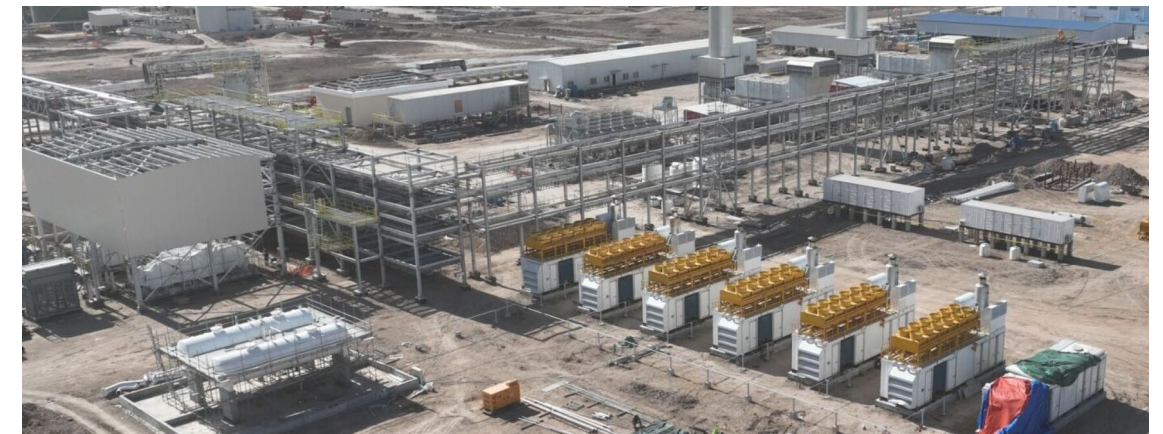
Rental Power Plant in KEBL
