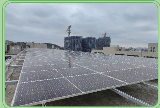
Photovoltaic System in the Factory Area
