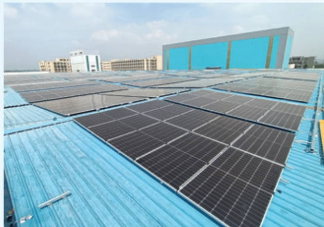
The Roof-mounted Distributed Photovoltaic (PV) Project of 179.58MW in Guli Key Industrial Park, Nanjing Jiangning Economic and Technological Development Zone
