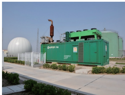
Joycome Biogas Power Generation Facilities
