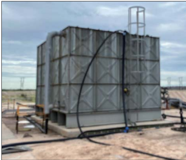
Figure 11-11 Mine water supply storage located directly above the portal
