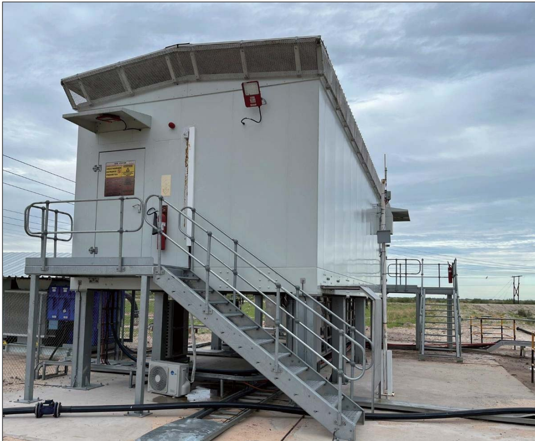
Figure 11-10 Boxcut located substation above the portal
