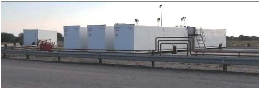
Figure 13-15 Fuel farm – Zone 5
