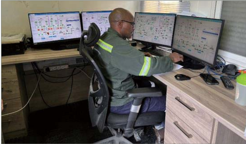
Figure 12-11 Process control room Source: KCM, 2023
