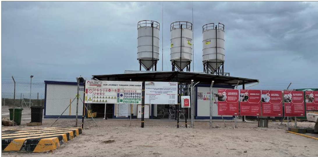
Figure 13-16 AECI explosives storage facility and detonator magazine Source: ERM, 2023
