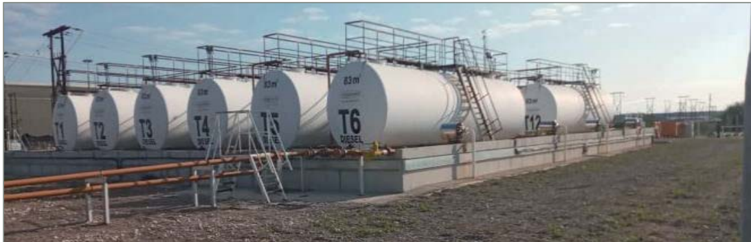
Figure 13-14 Fuel farm – Boseto processing plant
