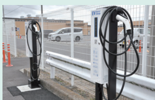
6 kW EV chargers
