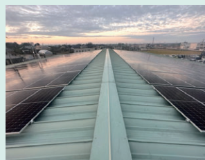
Solar panels on the roof of the hall
