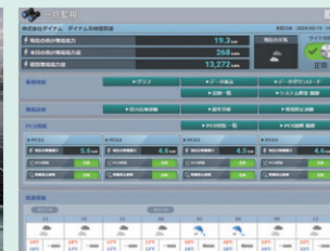
Display to manage the power generation by the solar panels on the roof of the hall
