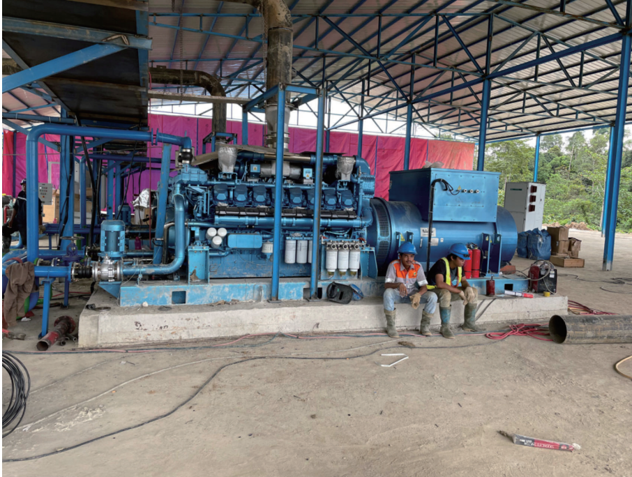
Figure 6: Power Generator Installed on Mine I Site
