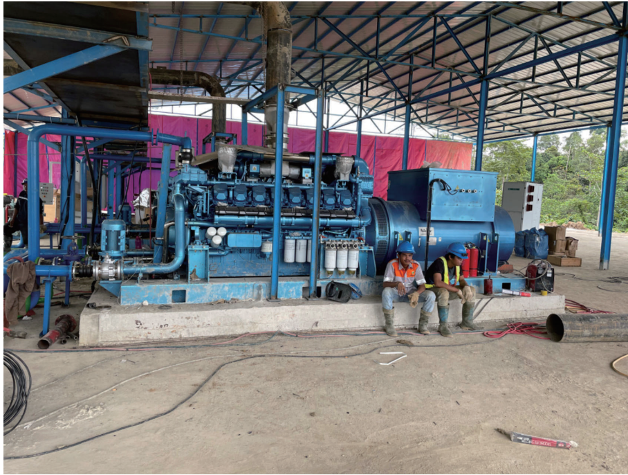
Figure 6: Power Generator Installed on Mine I Site
