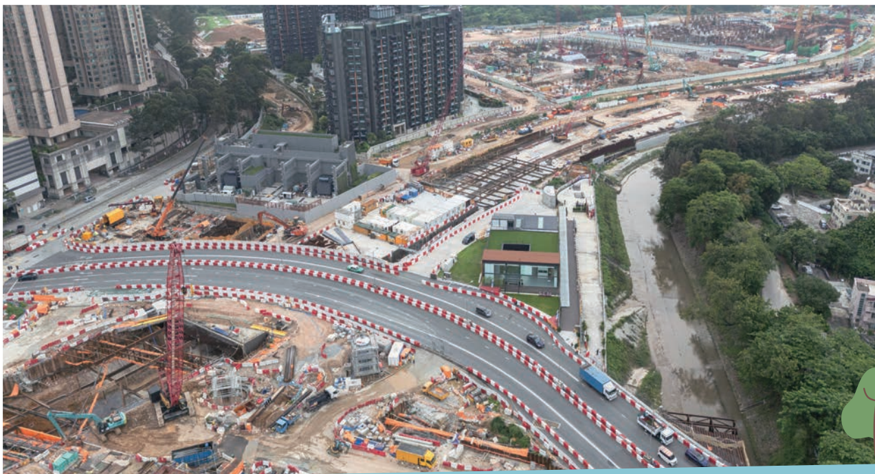
Fanling North New Development Area, Phase 1: Fanling Bypass Eastern Section (Shek Wu San Tsuen North to Lung Yeuk Tau) 粉嶺北新發展區第一階段：粉嶺繞道東段（石湖新村北至龍躍頭）
