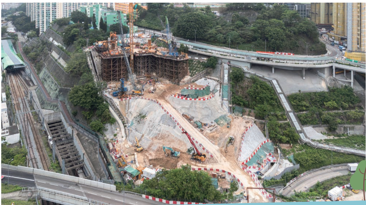
Site Formation and Foundation Works for Campus Expansion at Ho Man Tin Slope for the Hong Kong Polytechnic University 香港理工大學何文田斜坡校園擴建的地盤平整及地基工程
