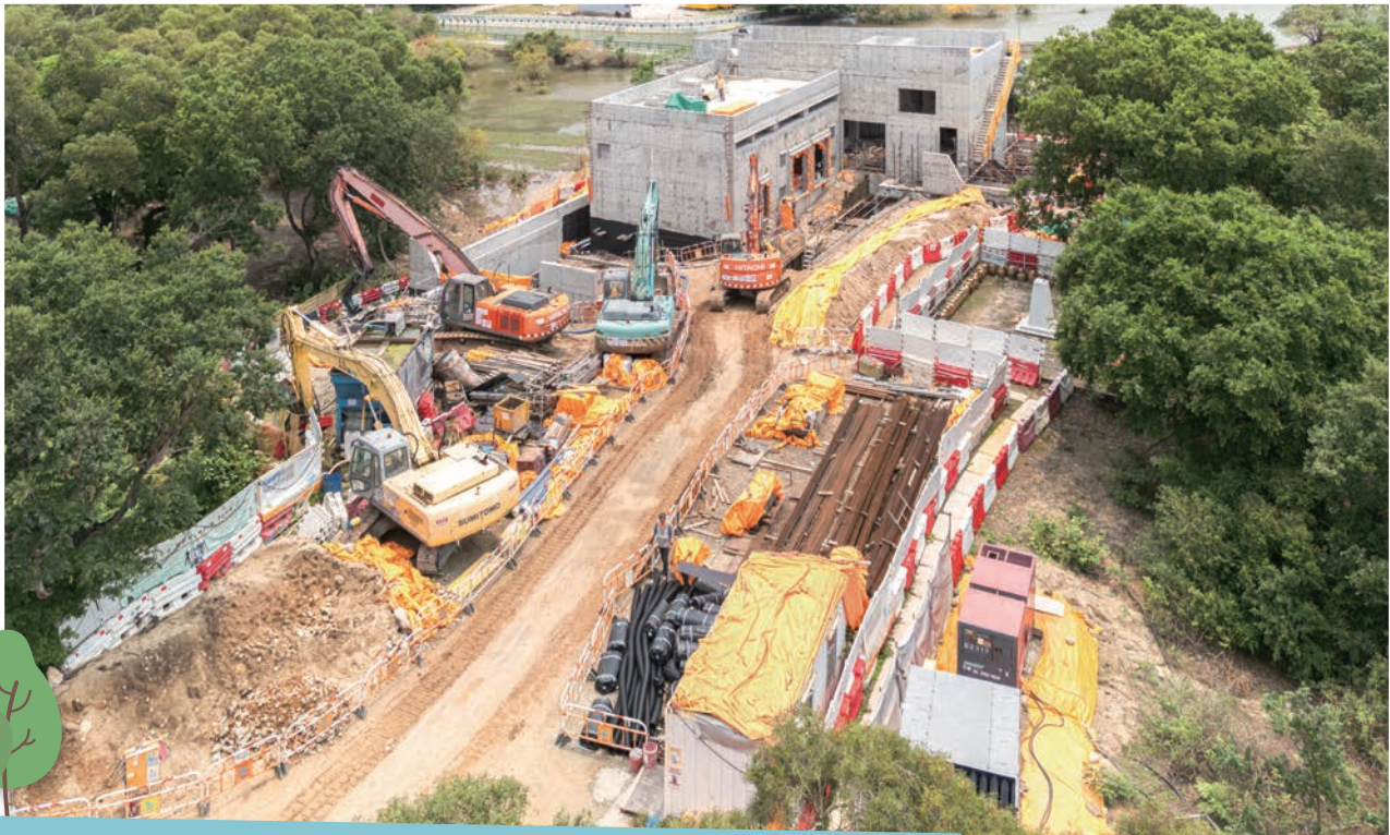
Upgrading of Pui O Raw Water Pumping Station and Pui O No. 2 Raw Water Pumping Station and Laying of Raw Water Mains along South Lantau Road 提升貝澳原水抽水站及貝澳二號原水抽水站及沿嶼南道敷設原水水管
