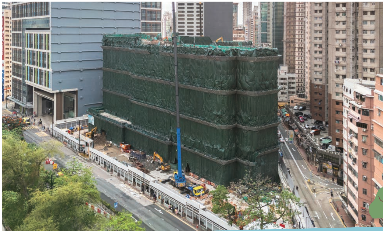
Demolition, Foundation, Superstructure and Associated Works Contract For Redevelopment of Kwong Wah Hospital (Phase 2) 廣華醫院重建計劃(第二期)的拆除, 地基, 上蓋建築及相關工程合約
