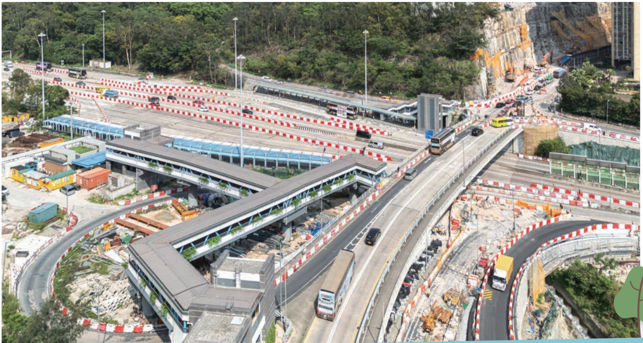
Development of Anderson Road Quarry Site — Road Improvement Works and Pedestrian Connectivity Facilities Works Phase 2A 安達臣道石礦場用地發展 — 道路改善工程及行人連繫設施工程第二期甲
