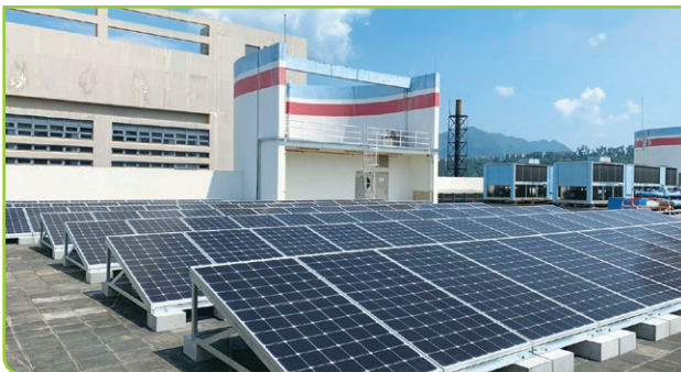
◇ The solar PV modules installed at the roof top of Lam Soon Building in Hong Kong 於香港南順大廈的屋頂所安裝的太陽能光伏組件
