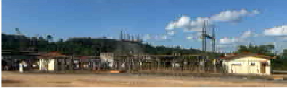
Figure 14-4: Main Transformer Station
