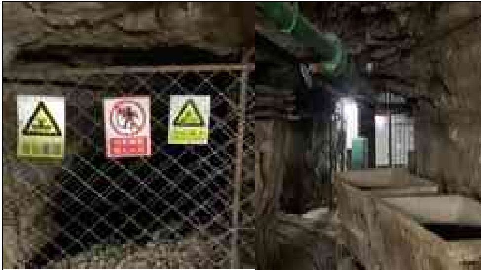
Figure 10-8: Photos of Level 5 Sump and Main Power Substation of Lianhuashan #5 Zone
