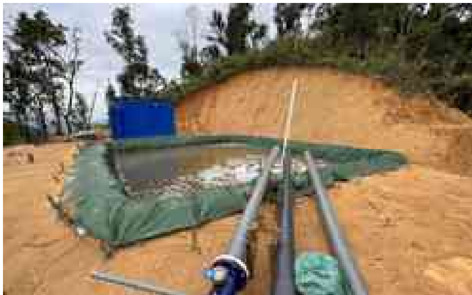
Figure 12-5: Leaching Solution Pond
