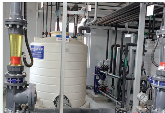
Waste Heat Power Generation Water Treatment Project
