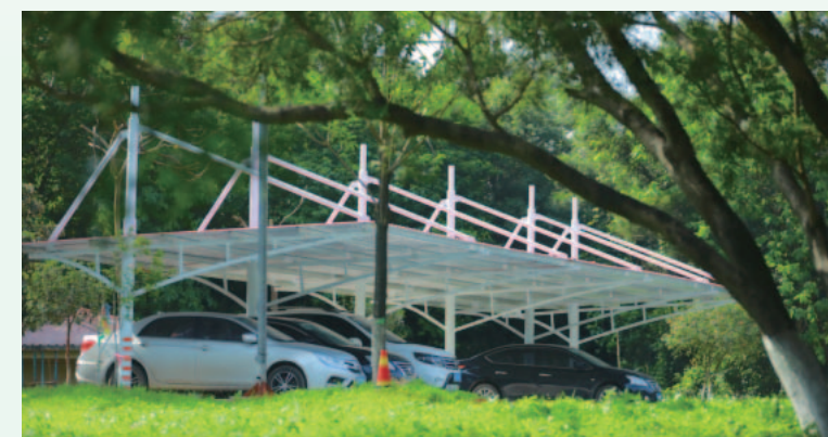
New Energy Carport
