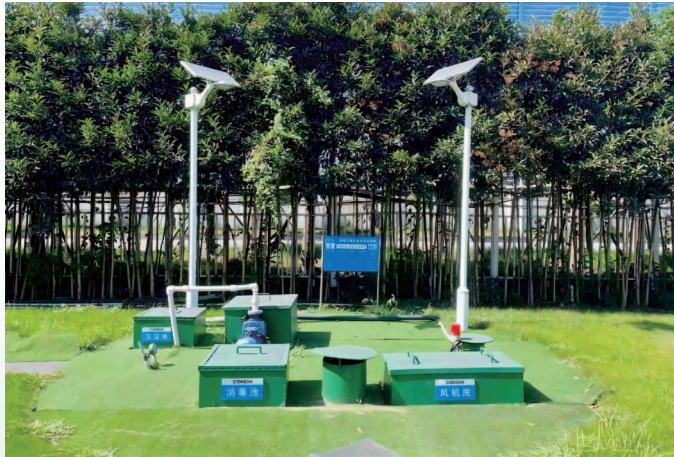
Yueqing Conch Sewage Treatment Facilities
