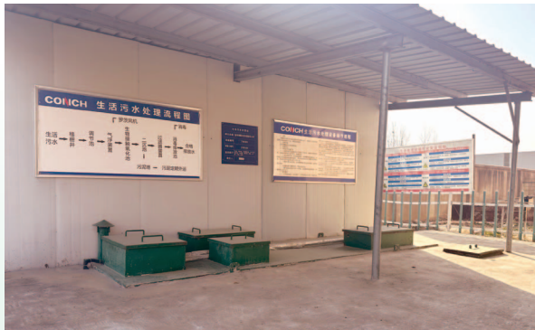
Domestic Sewage Treatment Station
