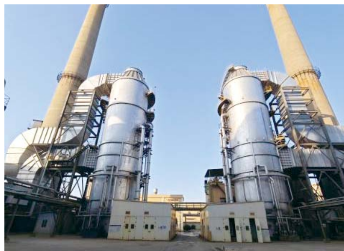
Wet desulphurisation technology reform
