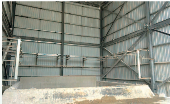
Dry-mist dust suppression at unloading port
