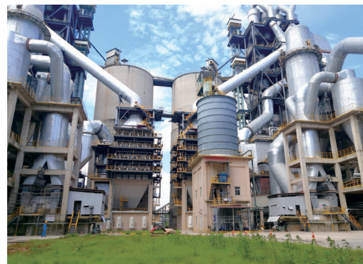
SCR denitrification technology reform
