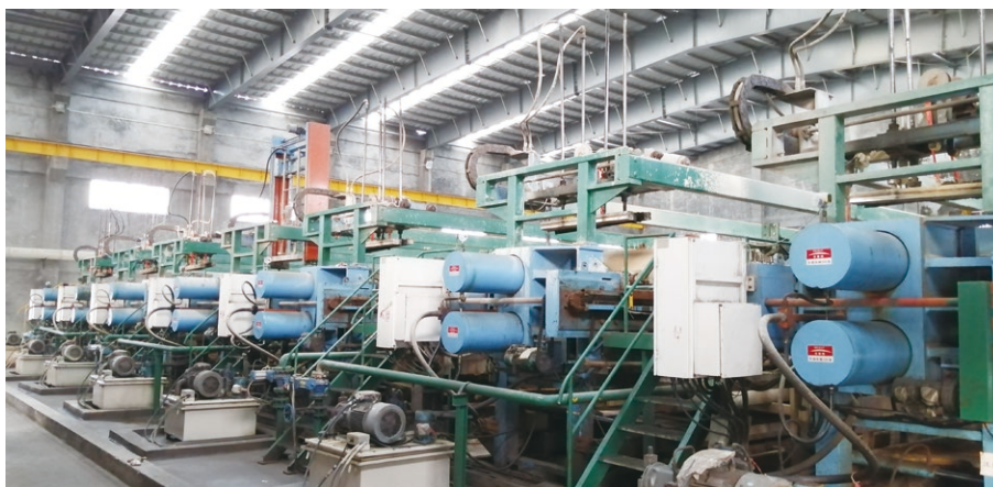
Sludge recycling equipment 污泥回收設備
