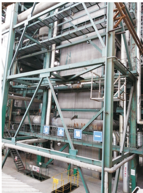
Circulating Fluidised Bed Boilers 循環流化床鍋爐
