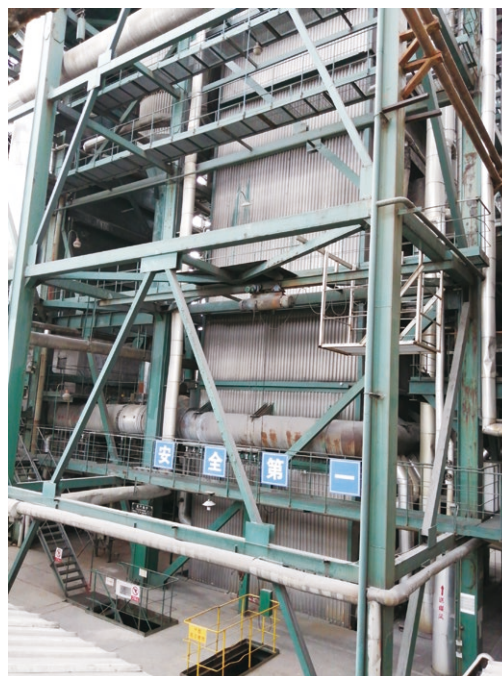
Circulating Fluidised Bed Boilers 循環流化床鍋爐
