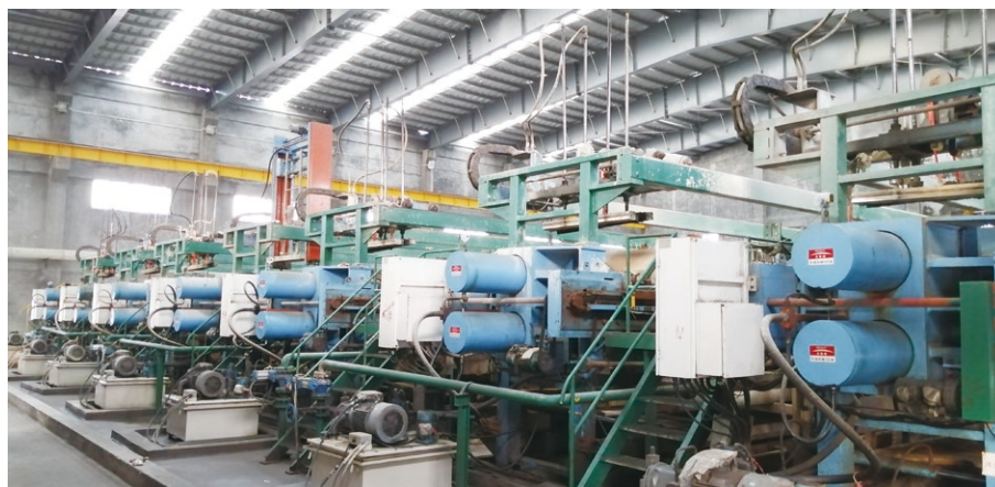
Sludge recycling equipment 污泥回收設備
