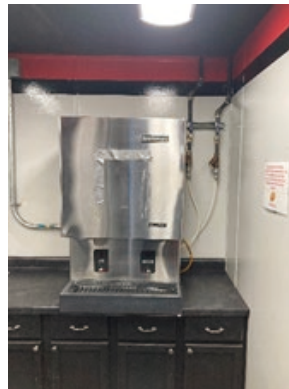
Photo from Ice Machine on Tower water
