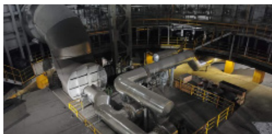
New exhaust system
