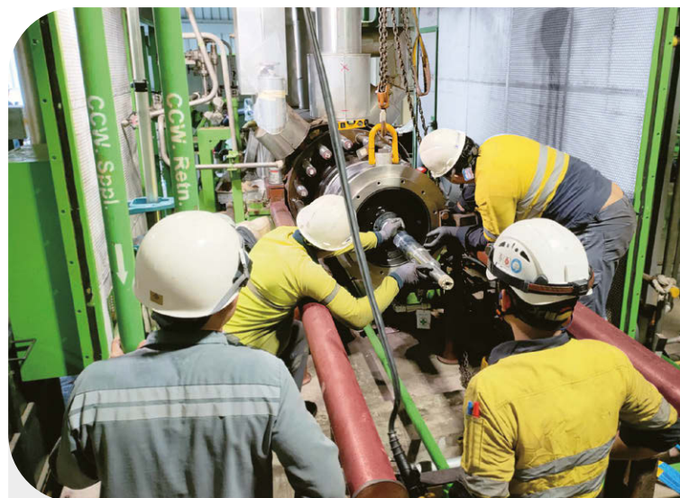
➤ RPCL technicians remove the cartridge on a boiler feed pump for enhanced reliability.
