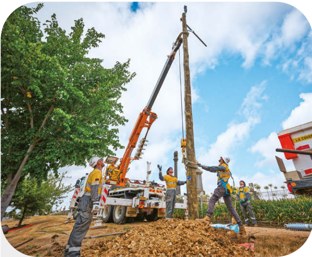
Powercor is advancing phase two of the Ballarat Network Upgrade, tripling the power capacity of Ballarat Base Hospital. The project will also support the local network to connect more rooftop solar and electric vehicles.
