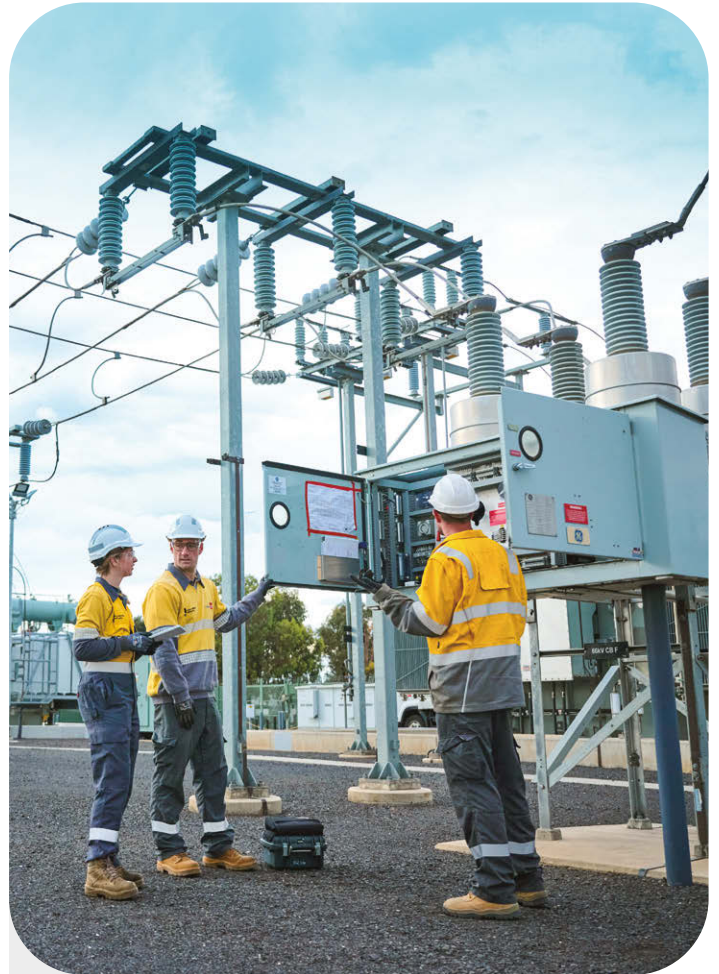
To prepare for an increased electricity demand over the summer period, United Energy upgraded 16 distribution substations to support over 2,000 customers in southeast Melbourne and the Mornington Peninsula.
