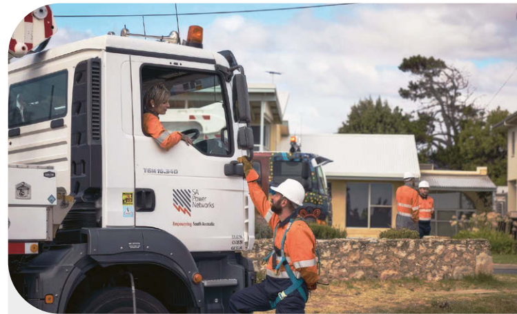
➤ An SAPN crew working in the Fleurier Peninsula, South Australia, where the company is carrying out the A$15.5 million Southern Outer Metro (SOM) Upgrade Project to enhance the reliability and capacity of its electricity network.
