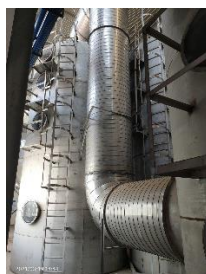
Spraying Tower for handling of paint exhaust
