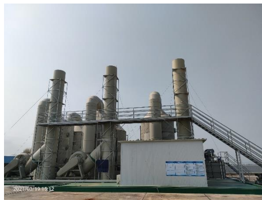
Acidic Mist Exhaust Treatment Facilities
