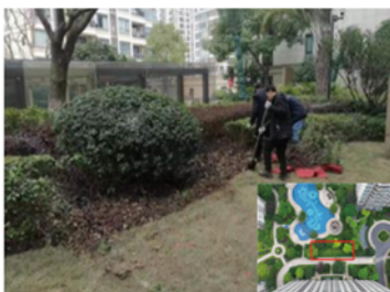
整改前 Before renovation
