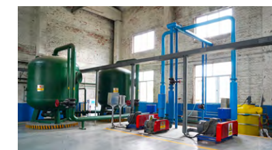
Wastewater Recycling Treatment of Sanshandao Gold Mine
