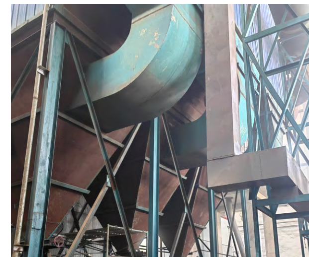
Dust Removal Facilities
