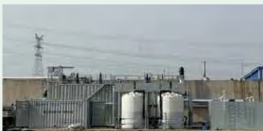
Demonstration Project for Improving Quality and Efficiency of Reclaimed Water Utilization
