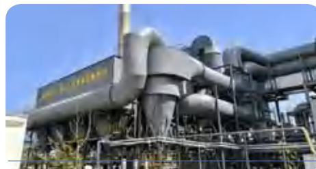
Integrated dry process for desulfurization, denitrification and dust removal utilizing catalytic ceramic fibre filter tubes
