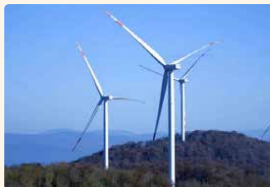
Senj Wind Farm Project in Croatia
