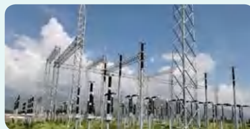
Ethiopia Power Transmission Project
