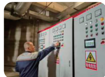
Adjust the Startup Mode of the Air - Conditioning Host
