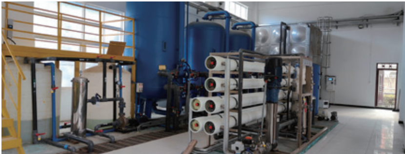
Zero-discharge Wastewater Project of Midu Cement
