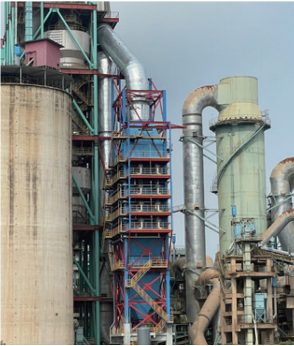
Ultra-low emissions transformation equipment of Nanning Cement
