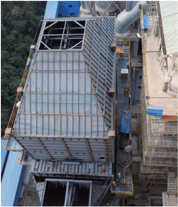
Dust and nitrate integration removal equipment in Anshun Industry Park
