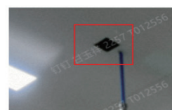
3. Production workshop environment not properly sealed
