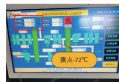
6. Dehumidifier dew point is set too low.
