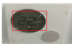
2. Air conditioning temperature is set too low
