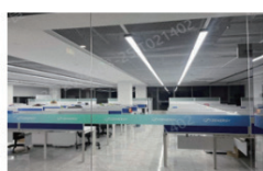
1. Office lighting left on when unoccupied
