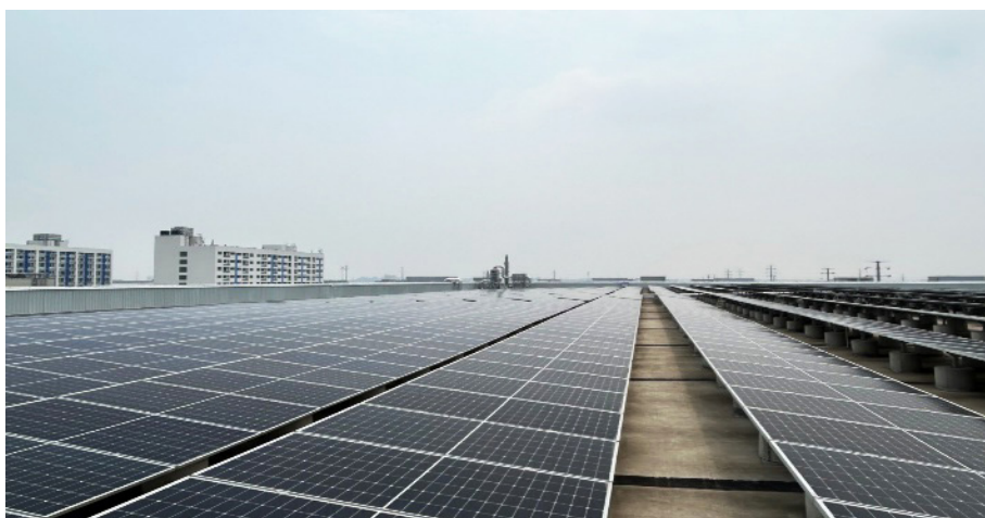
4.2MWh of new power generated by installation of rooftop photovoltaic in Zenergy's production base
