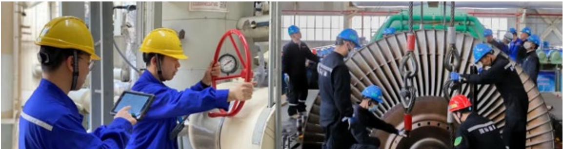
The thermal power plants in Beijing underwent a comprehensive "health check" to prepare for "riding out the summer peak"
