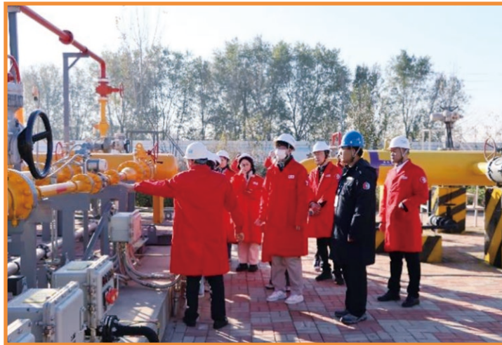
Media Tour Visiting China Gas Tianjin Jinghai High-Pressure Transmission and Distribution Gate Station
