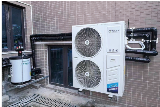
Pilot Projects for Household Underfloor Heating Units
