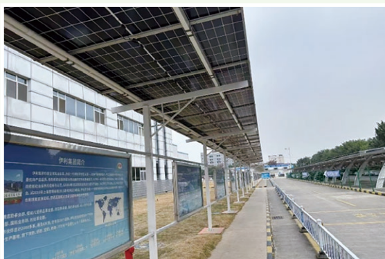
Yili ASEAN Distributed PV Project in Nanning
