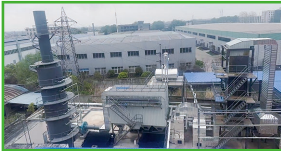
Biomass clean heating plant of Youfang Town New Materials Industrial Park in Yangzhong
