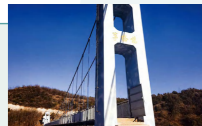
Construction of “Happiness Road” Bridge in Maota Village, Xiangkou Township, Yunxi County by Hubei Company
