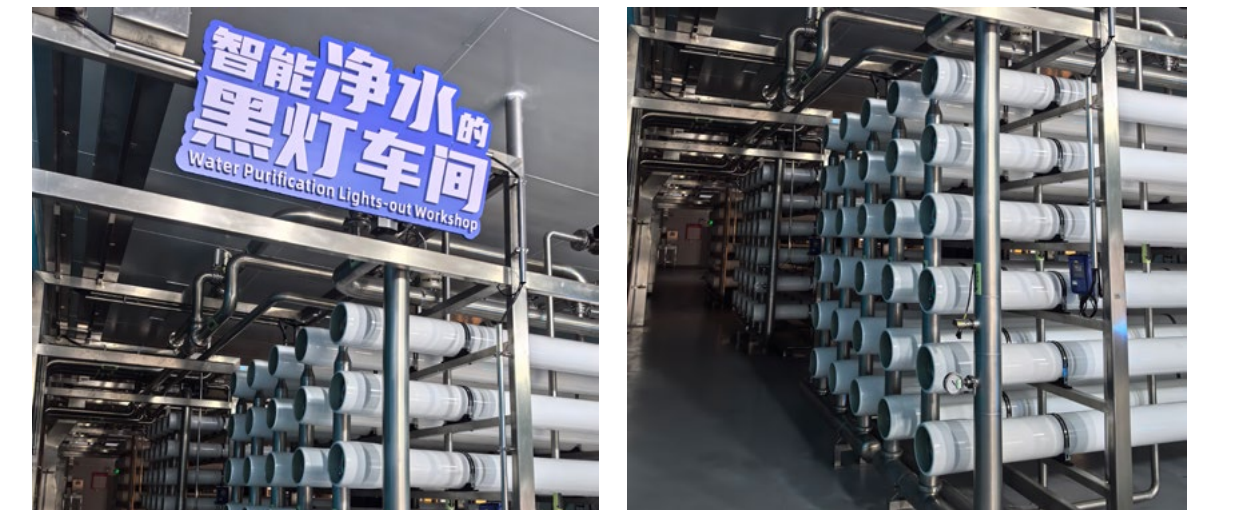
Haitian water treatment workshop
