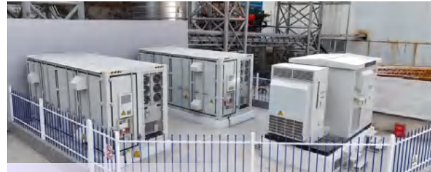
▶ The energy storage power plant at our Chinese processing facility.
