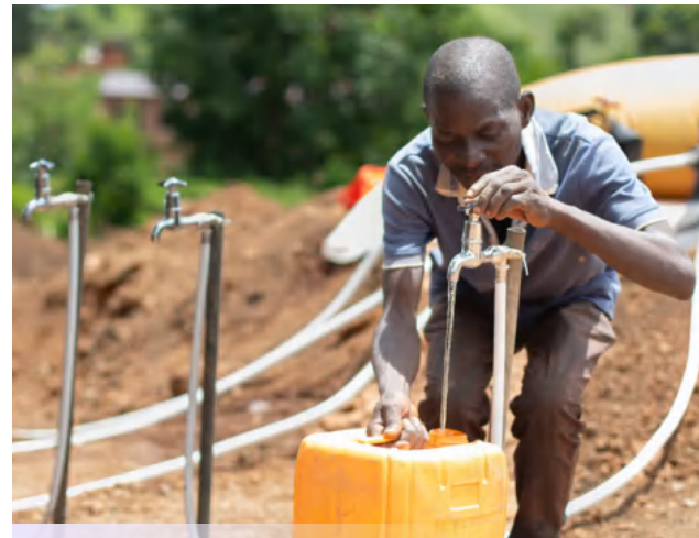
▶ In February 2025, TFM and UNICEF supported the Manomapia community in the fight against cholera by providing essential supplies, installing four 6,000-liter water tanks, and deploying water trucks to ensure safe drinking water.
