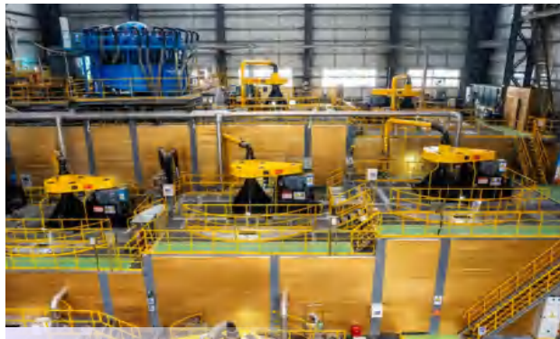
▶ An odor-free, dust-free mineral processing plant at CMOC China
