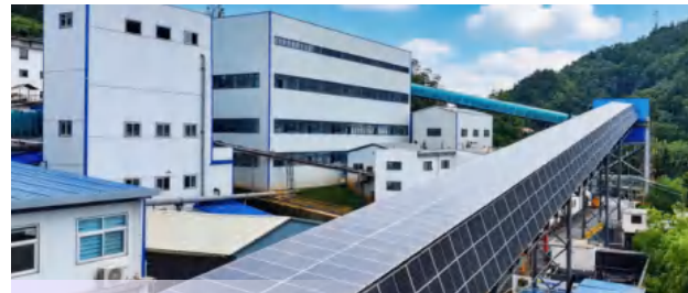
▶ Distributed photovoltaic system at CMOC China
