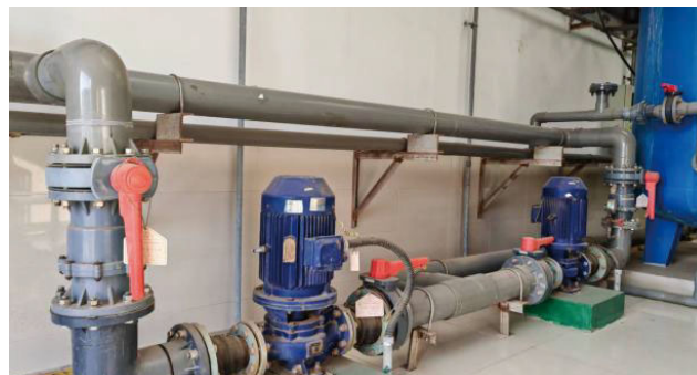
Clear Water Pump Conveying Device of Tongzhou Company
