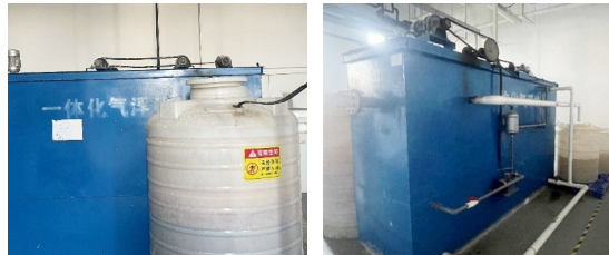
Wastewater Treatment Facility at Jiangmen Base
