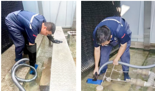
Optimization of Cooling Tower Cleaning Model at Jiangmen Base
