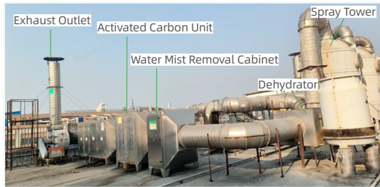
Upgraded Waste Gas Treatment System
