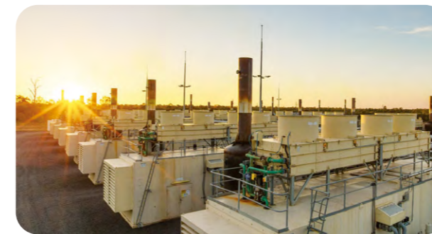
EDL's 64 MW Moranbah North Power Station located in Queensland, Australia
