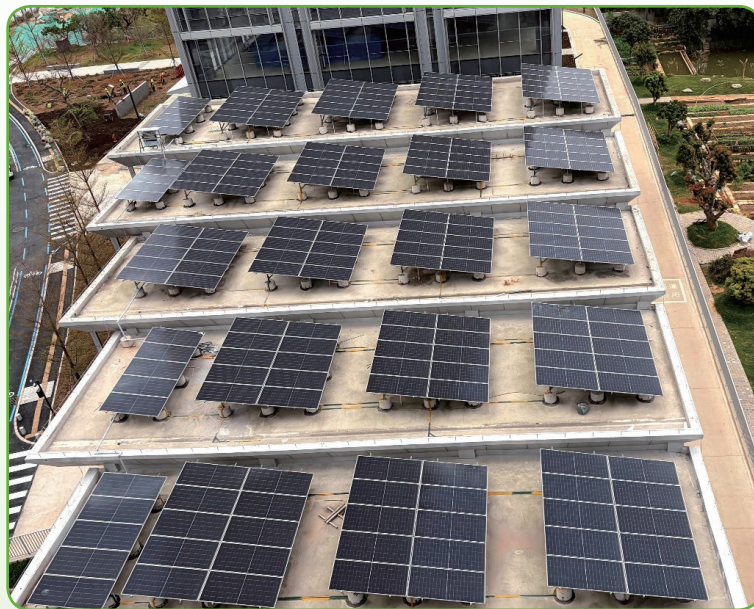
The fourth phase factory building's rooftop photovoltaic project 四期廠房屋面光伏項目
