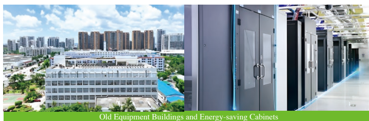
Old Equipment Buildings and Energy-saving Cabinets
