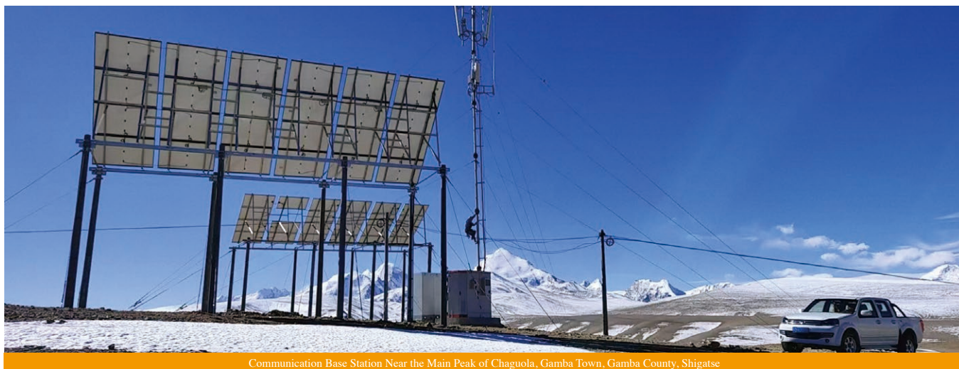
Communication Base Station Near the Main Peak of Chaguola, Gamba Town, Gamba County, Shigatse
