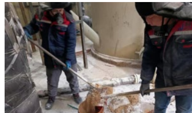
Cover leaked liquid with sand and soil
