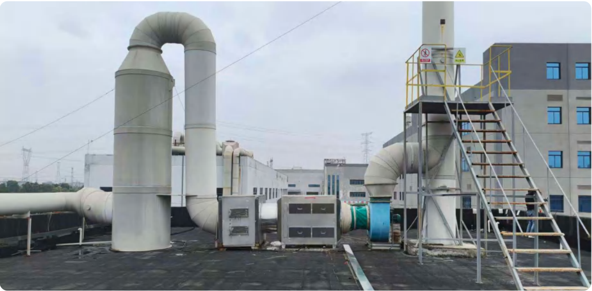
Renovated Exhaust Gas Treatment System (two-stage activated carbon adsorption) for the Hazardous Waste Storage Area
