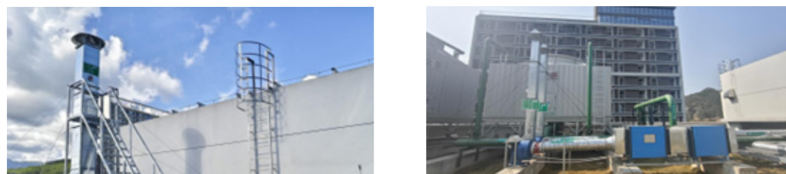
Exhaust Gas Treatment Facility in the Factory
