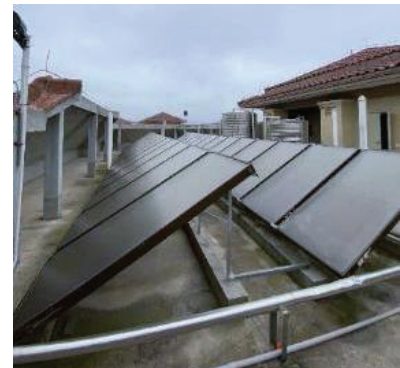
Solar water heating system
