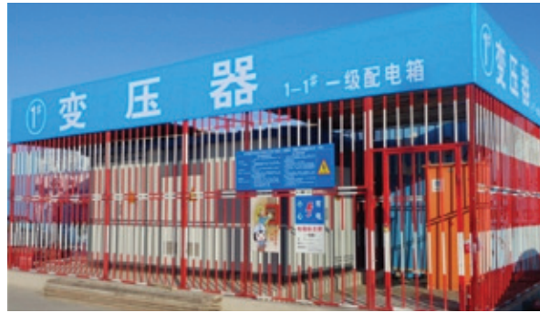
Protection for box transformer
