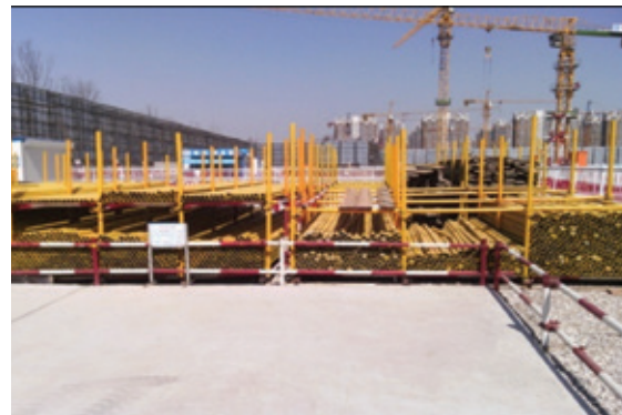
Material stacking rack
