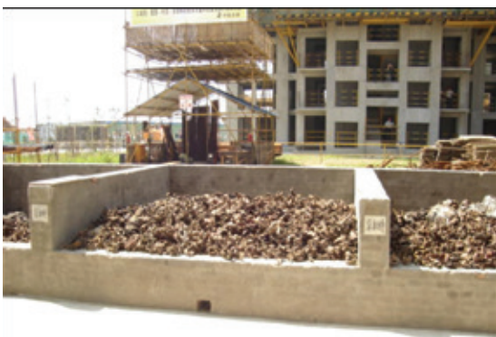
Material recovery tank
