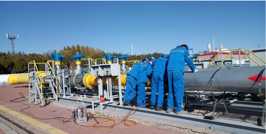
PICC P&C provided special disaster prevention and loss prevention risk survey services for the Central Asia Natural Gas Pipeline Project
