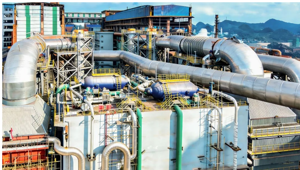
World's First Commercial Supercritical Carbon Dioxide Power Generation Unit "Super Carbon One"
