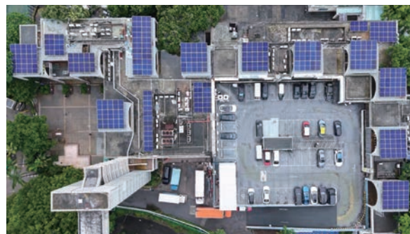
CR Power's 150kWp Distributed Photovoltaic Power Project at Sui Wo Court in Hong Kong, the first pilot project for renewable energy cooperation between CR Power and Emperor International, achieved full-capacity grid connection in August 2025
