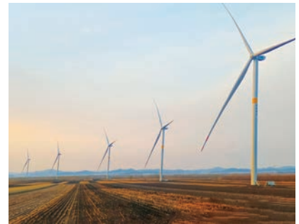
In April 2025, the Heilongjiang Huanan 300MW Wind Power Project achieved full-capacity grid connection
