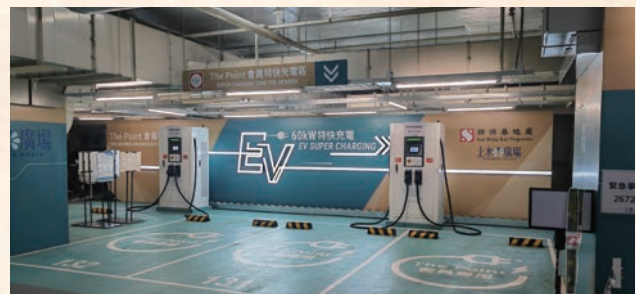
Sun Hung Kai Properties Landmark North Charging Pile Project
