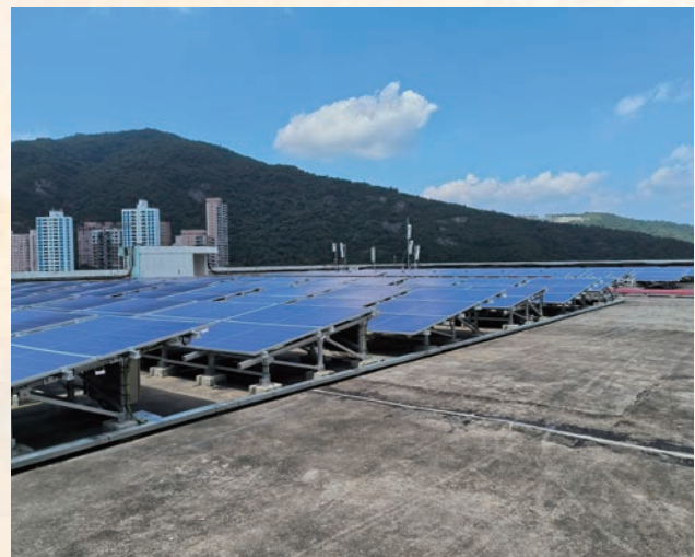
The 720kWp Distributed Photovoltaic Power Project by China Resources Logistics, located in Shatin District, Hong Kong, marks CR Power's first Hong Kong-based project. Since June 2020, the project has generated an average of 670,000 kWh of clean electricity annually
