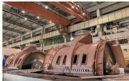
Comprehensive efficiency improvements and transformation for Unit #2 at Hezhou Power Plant
