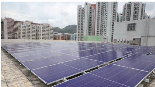
CR Power's 180kWp Distributed Photovoltaic Power Project at East Asia Industrial Building in Hong Kong achieved full-capacity grid connection in August 2025
