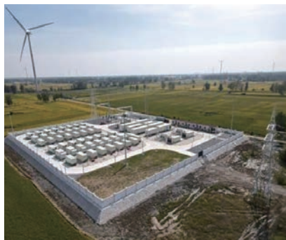
In November 2023, the 200MW Shangtang Wind Power Project at Anhui Fengtai Base achieved full-capacity grid connection
