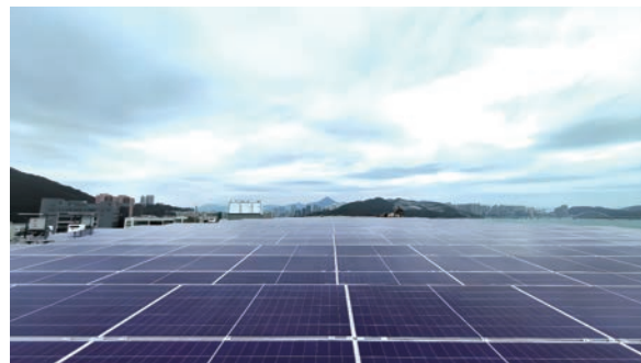
CR Power's 480kWp Distributed Photovoltaic Power Project at China Resources Logistics' Chai Wan Warehouse in Hong Kong achieved full-capacity grid connection in October 2025
