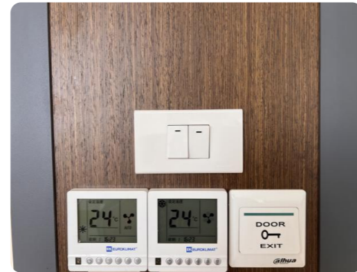
Office air conditioning uniformly set to 24°C
