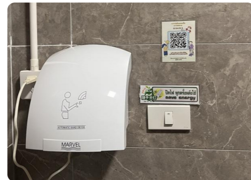
Sign for turning-off lights after use
