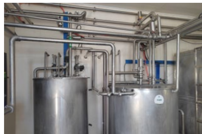
· Retrofit of Combined Cleaning for Dairy Parlor Equipment ·
